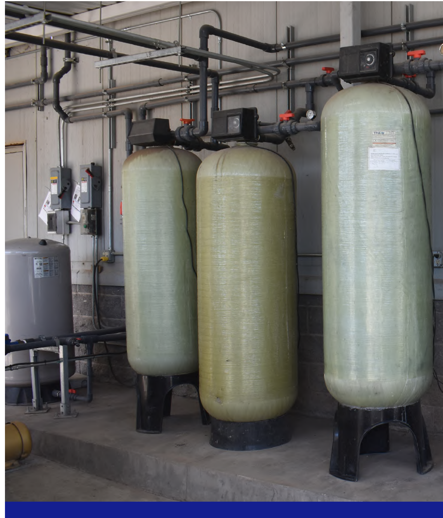
Reverse osmosis treatment in Mexicali, SunPower Mexico
