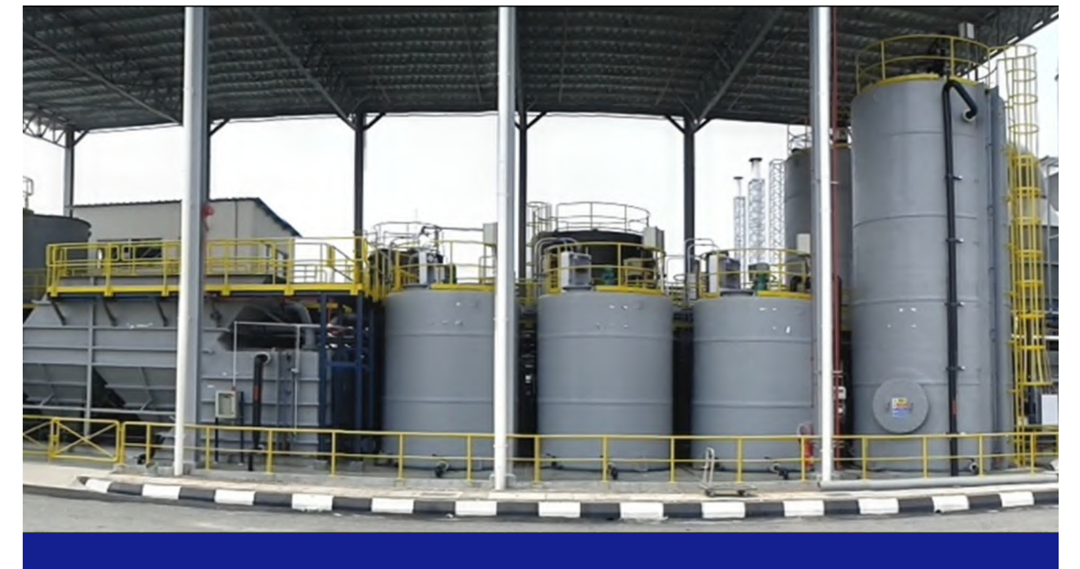
Fluoride Waste Treatment Plant in SunPower Malaysia
