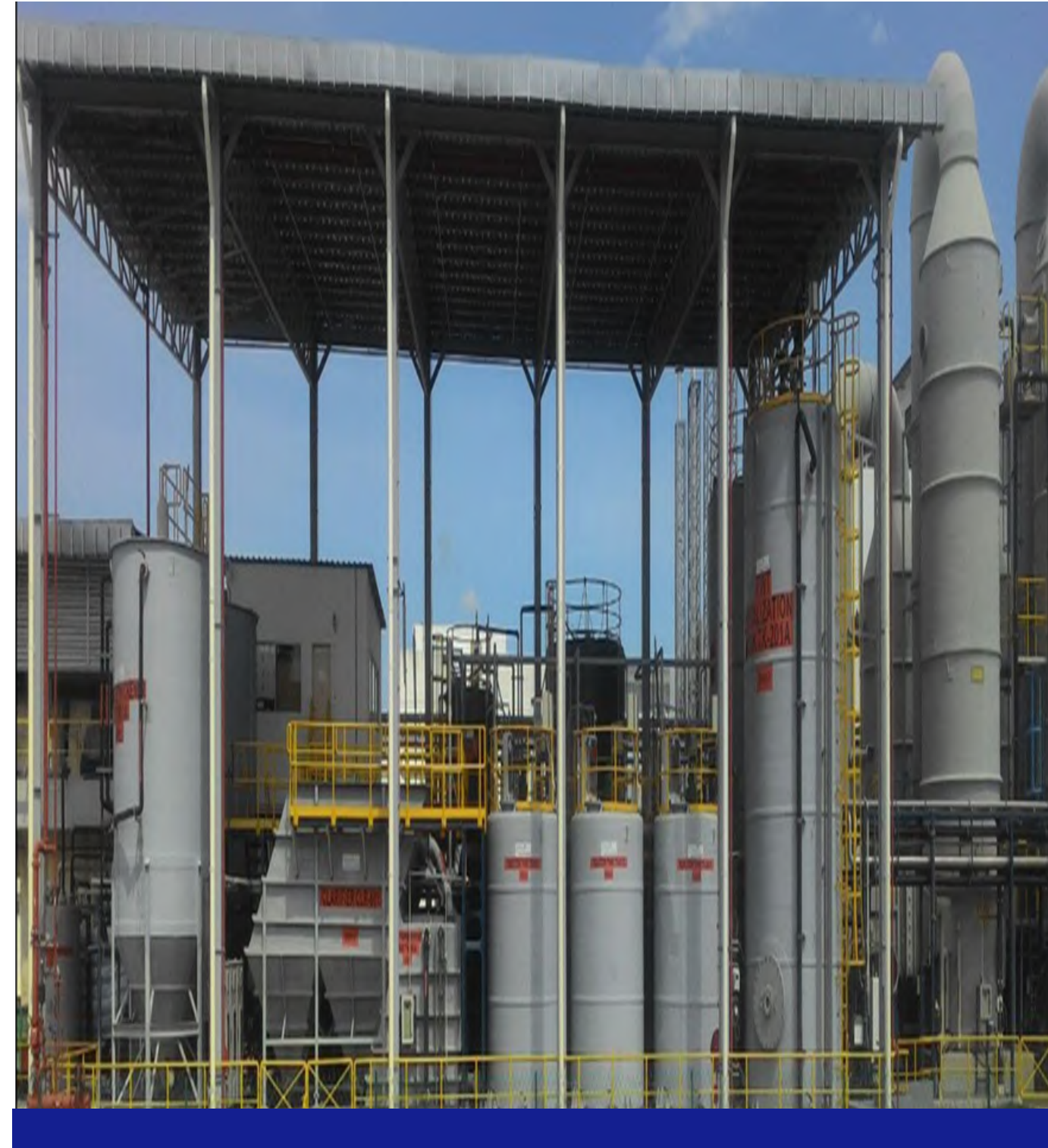
Wastewater Treatment Plant in SunPower Malaysia
